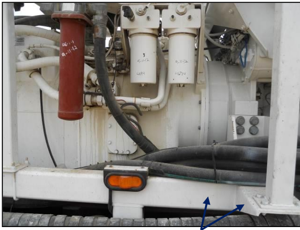
Picture 1: Mounting Location (Tie-in Surfaces)
